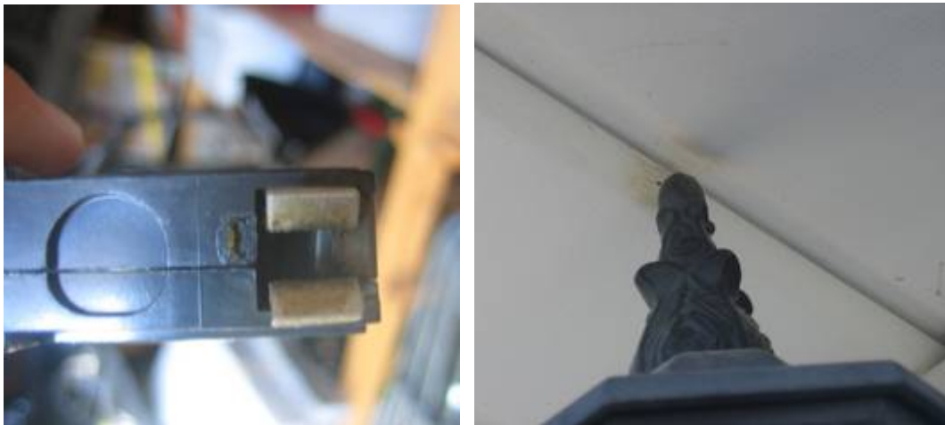
Photos 4 & 5: Burn Marks on Circuit Breaker and Outdoor Lighting
