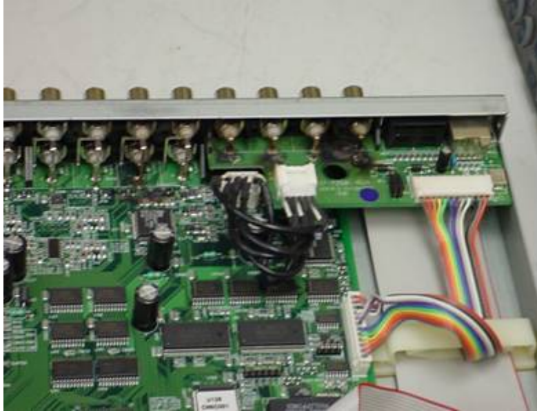
Photos 4: Burn Marks on Multiplexer Inputs
